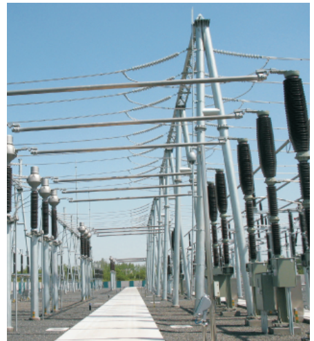
110kV current transformer operating in Yangzhou station
