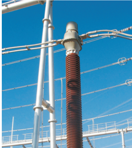
363kV current transformer in operation
