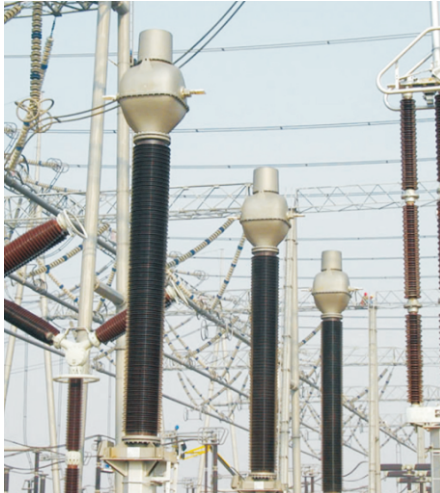
550kV current transformer in operation
