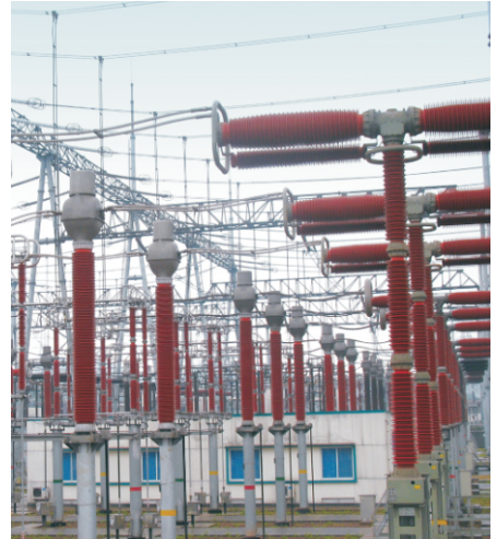
550kV current transformer operating in Yibin, Sichuan
