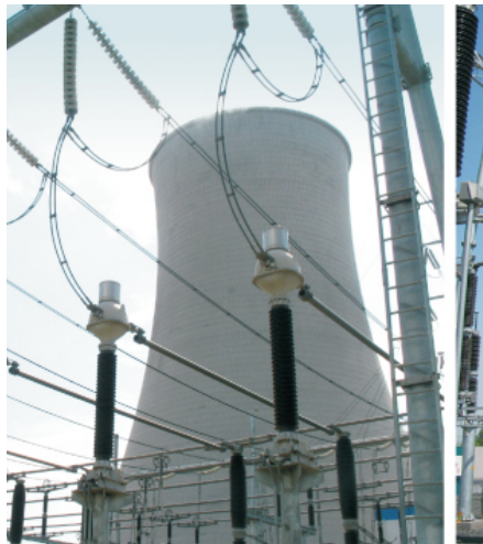
220kV current transformer operating in Huaneng Changchun Power plant
